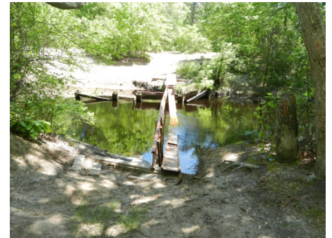
Ruins of a recently constructed illegal and dangerous foot bridge across Great Egg Harbor River, about 120 feet from the Blue Hole. The river is not tidal at this point. The water appears tea-colored because of cedar and bog iron in the area. Not to worry ... it is all natural!
